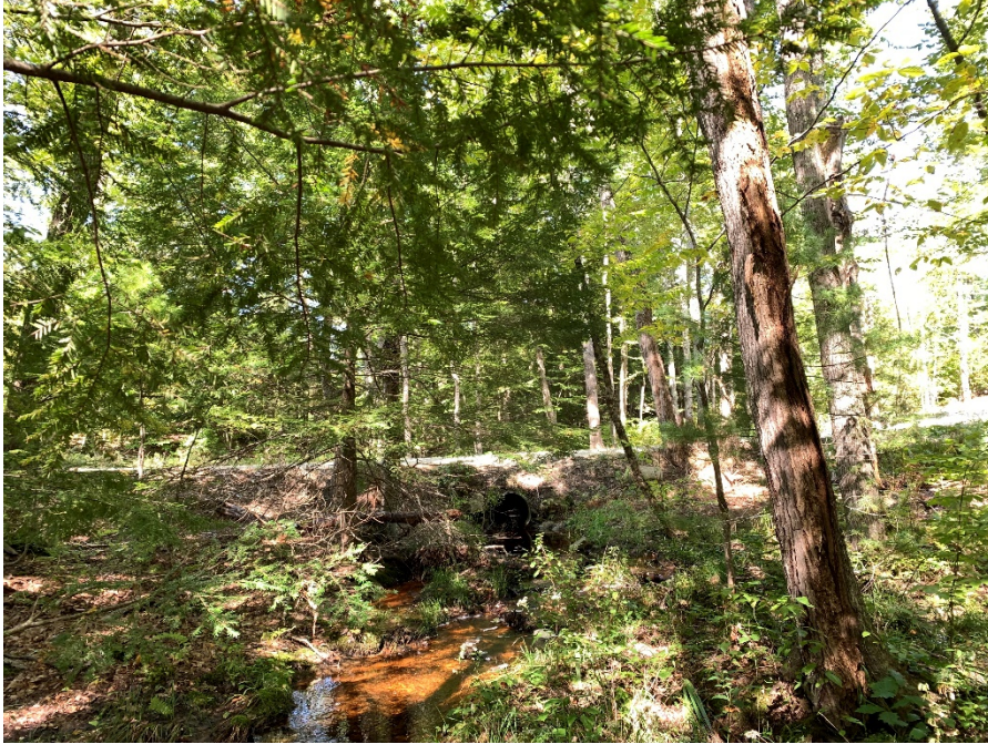
Photograph No. 9: Looking easterly into the Wetland 7 and existing culvert at Jamps Trail.
